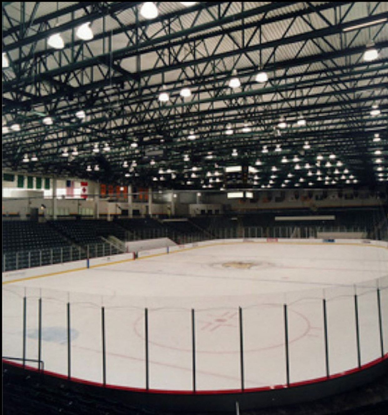
Metal Halide Fixtures at Berry Events Center, Northern Michigan University. [www.holophane.com]
